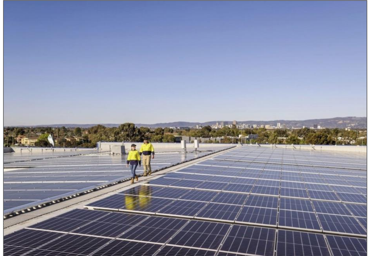
Ikea Adelaide's 1.2 MW rooftop solar array will be coupled with a 700 kW carpark and 3.45 MWh battery.
